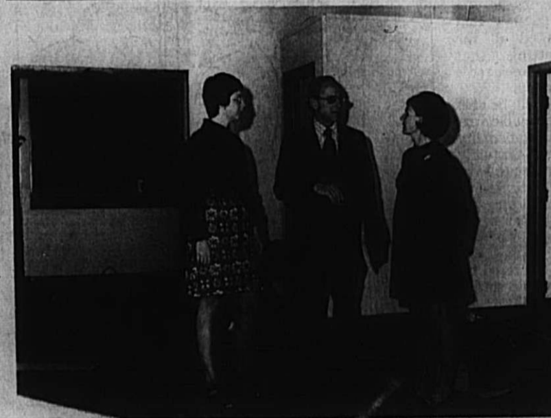
EXAMINE RENOVATION PROGRESS—Robert B. McNamara, vice-president of the St. Mary's Child Center board of directors, discusses the current renovation project underway at the center with Mrs. Lawrence Kennedy, right, board member, and Miss Kathleen Kell, caseworker. The Child Center, a member agency of the United Way which provides professional services for children with special needs, will receive the proceeds of the 11th annual Benefit Dinner to be held Thursday, Nov. 1, at the Indianapolis Athletic Club. McNamara is serving as co-chairman of the event with Mrs. George Schnieders. Tickets are $50 per person and are available from the co-chairmen.
