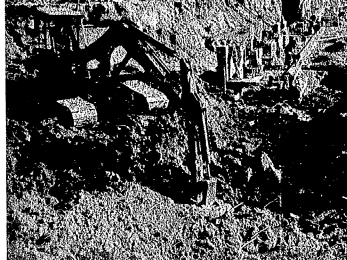
CONSTRUCTION PROGRESS—Shown above is the excavation and foundation work underway at the new St. Augustine's Home for the Aged, 2200 W. 86th St. in northwest Marion County. Announcement of a surprise grant of $700,000 this week will enable the home's capacity to be enlarged by 20 per cent.
